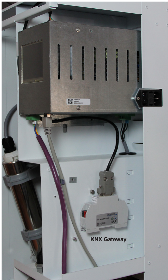
Fig. 1: KNX gateway installed
