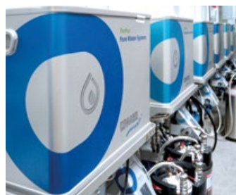
Multi-stage water treatment for high-pressure humidification
