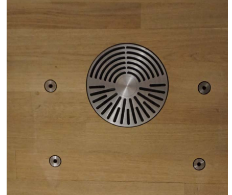
During a concert, each of the 2,100 seats is supplied with draught-free supply air via a combined swirl/swirl diffuser
