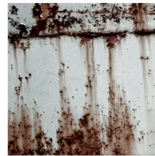
Protection from rust and corrosion
