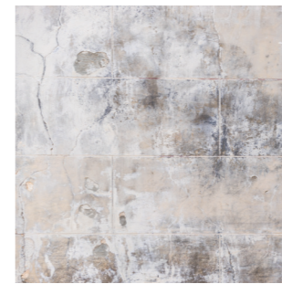
Preventing mold and rot
